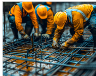
Increasing the cross section, building structure reinforcement, and planting steel bar framework
