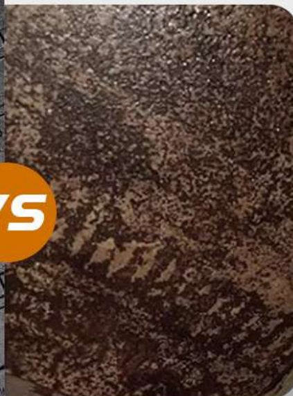
Shallow penetration Rust transformation superficiality
