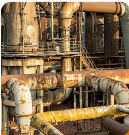
Chemical plant pipeline
